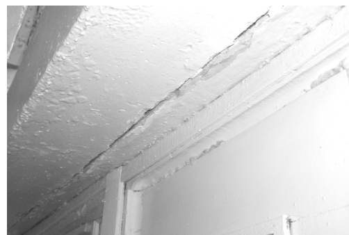
Fig. 1. Vertical and diagonal cracks and other defects in walls
