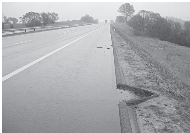
Fig. 5. An example of storm water runoff directive system on the Vilnius–Klaipėda highway (Lithuania)
