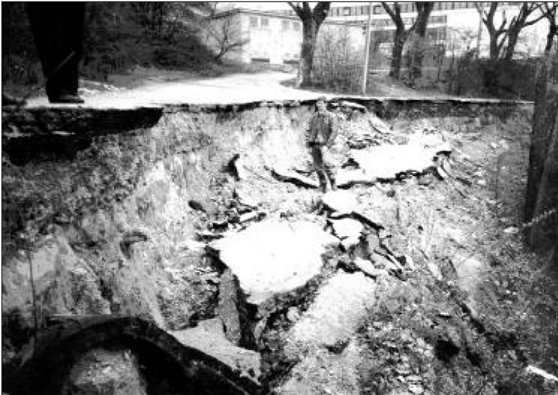
Fig. 4. Landslide developed in Slėnio street, Kaunas city, 1996 (photo by V. Marcinkevičius)
