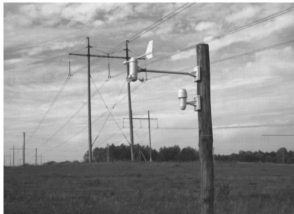
Fig. 1. High-voltage transmission lines with devices for measurement of meteorological parameters.
